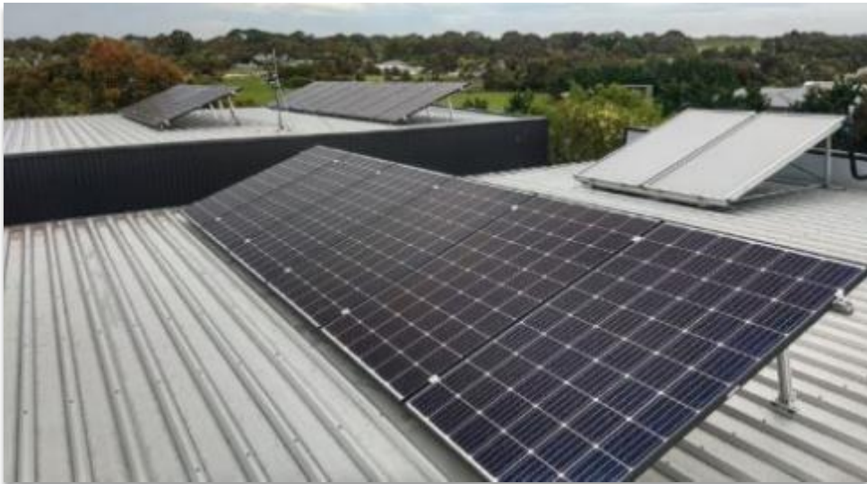
Traditional – externally applied roof PV
