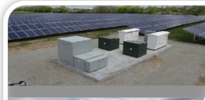
Energy Storage - Solar Hybrid Project
