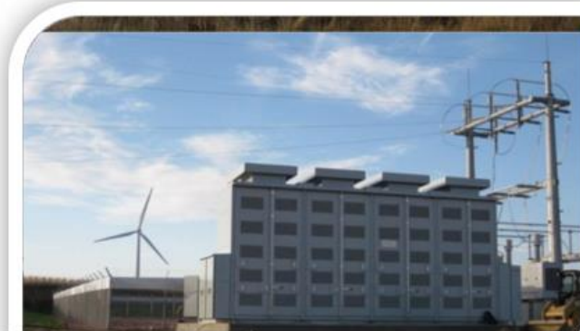
Energy Storage – Wind Hybrid Project
