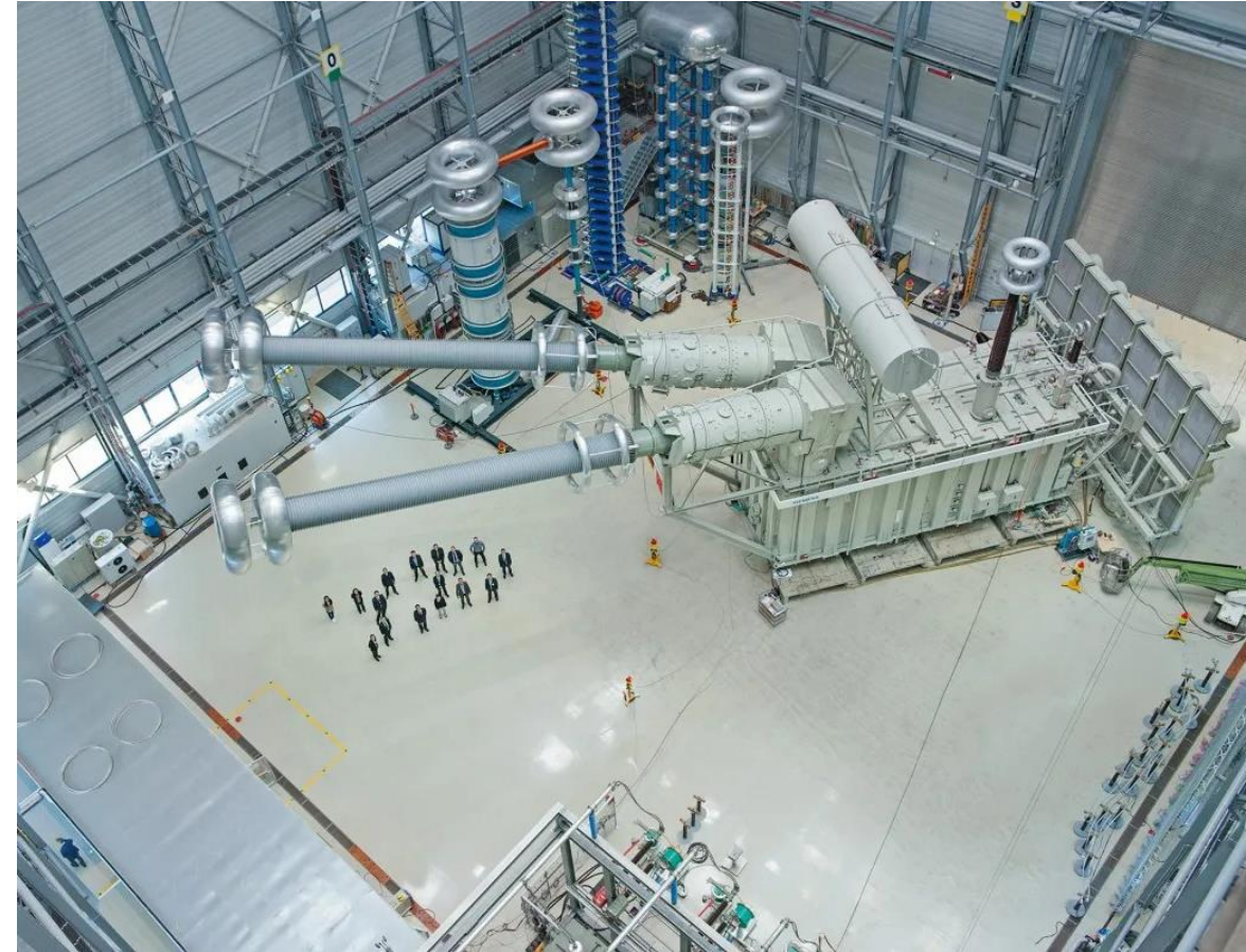
World's first 1,100 kV HVDC transformer
