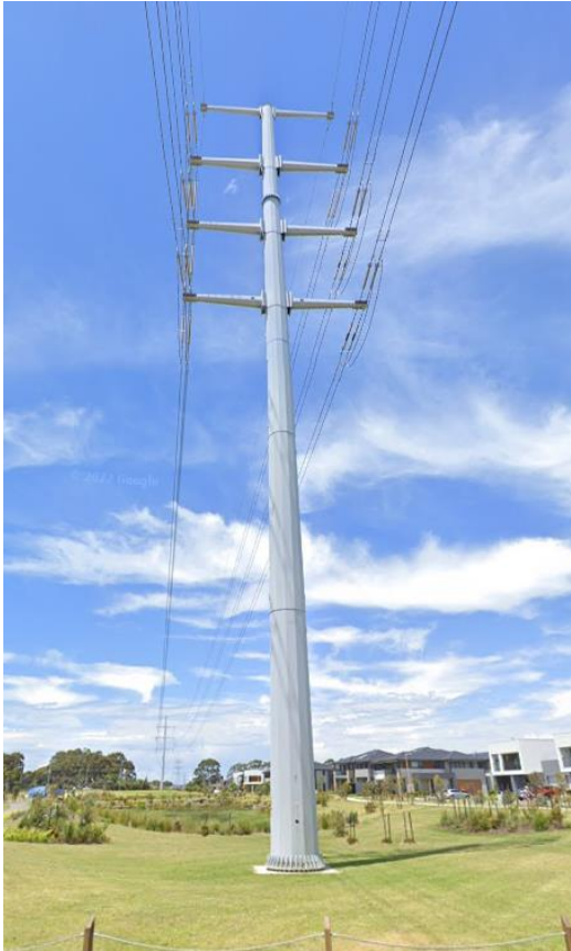
Steel Pole for EHV
