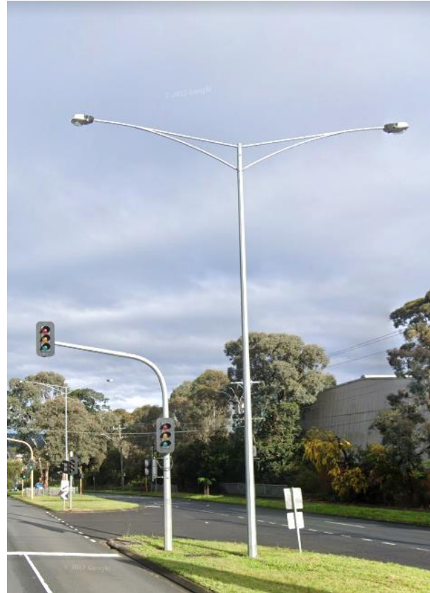
Steel Pole for Street Lighting
